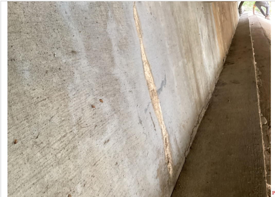
Abutment cap 1 Hairline cracks w/ leaching (Typical abutment 2)
