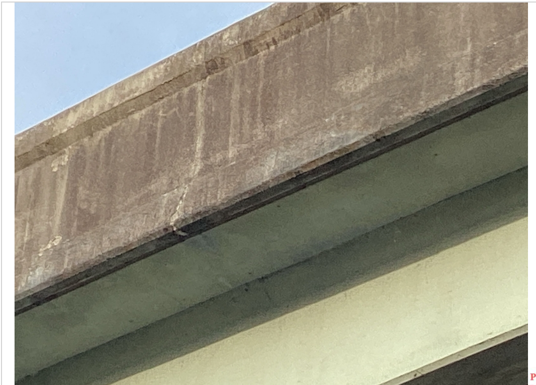
Span 2 Right bridge rail - Hairline cracks with leaching
