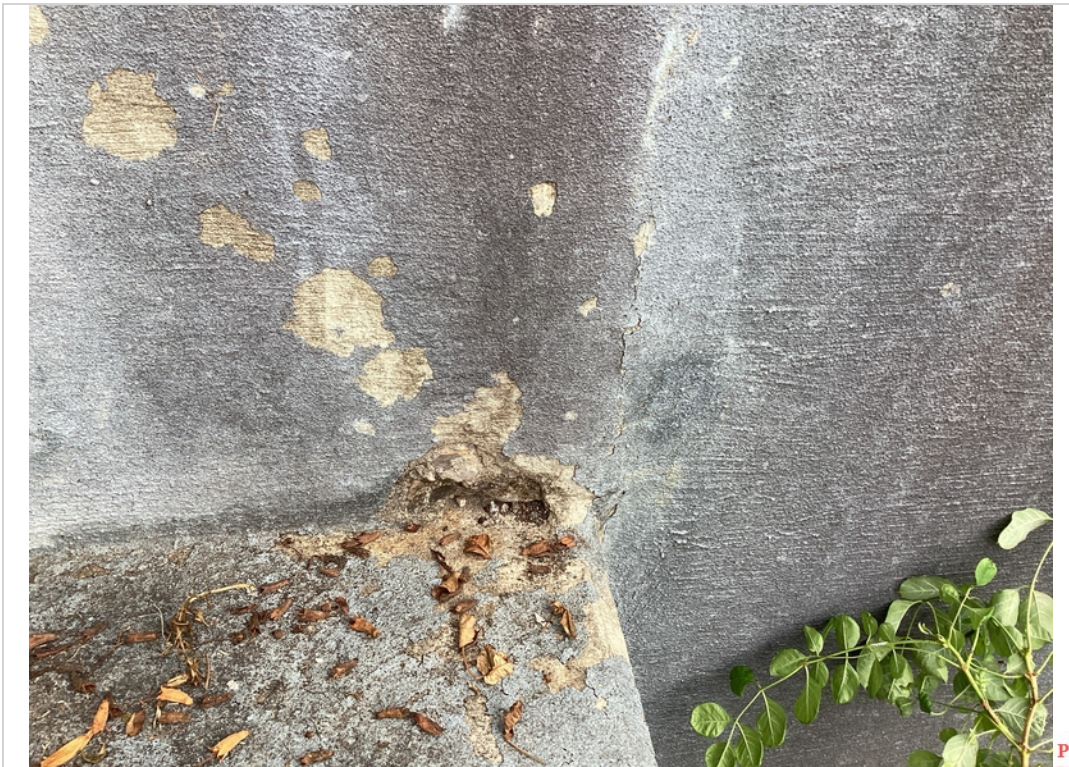
Wing 2 left - spall (4"diameter x 2"D)
