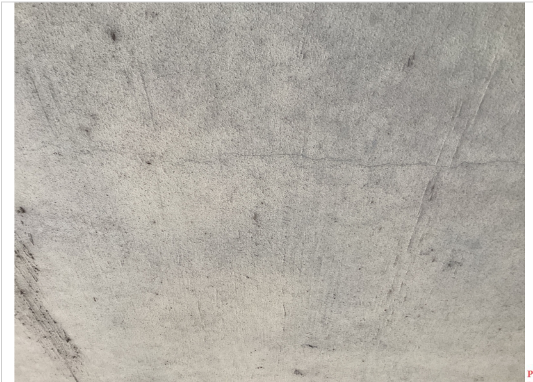
Span 1 left overhang - Hairline cracks
