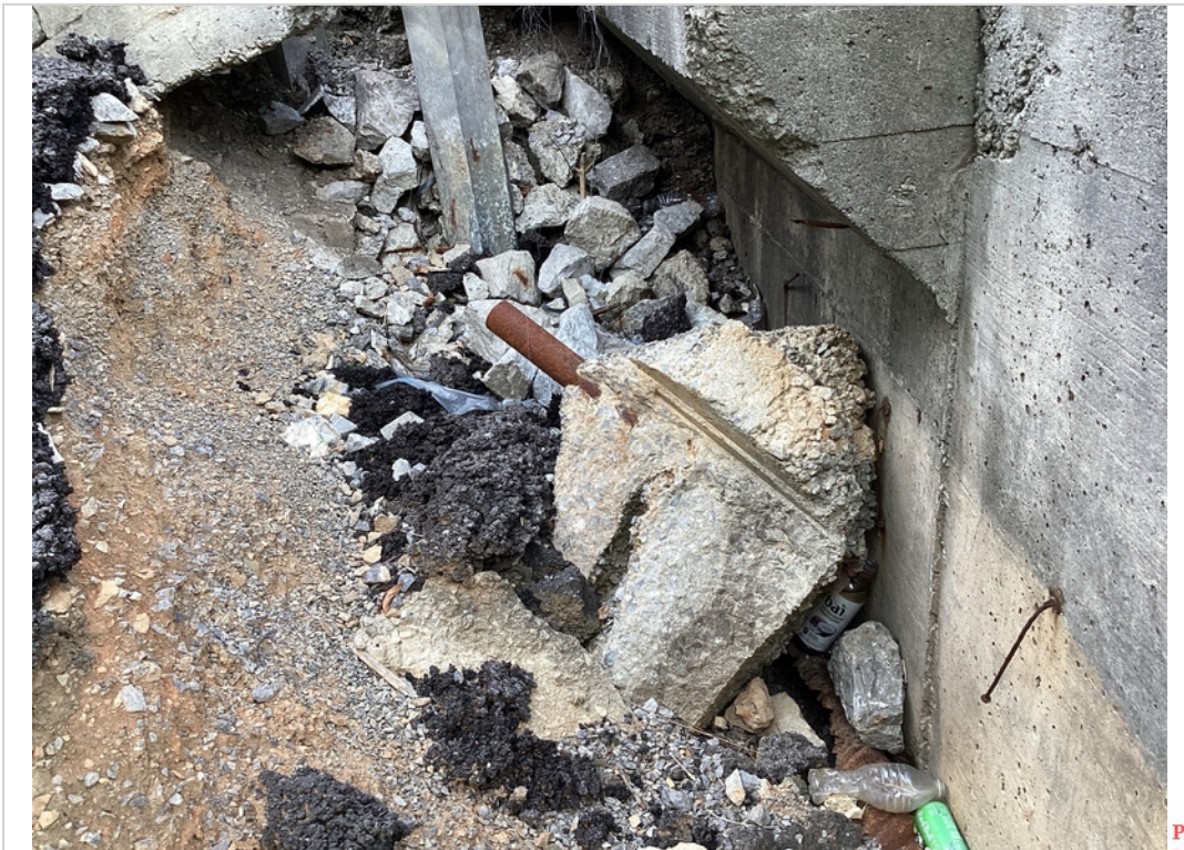
Approach 1 right embankment and drain pipe - erosion
