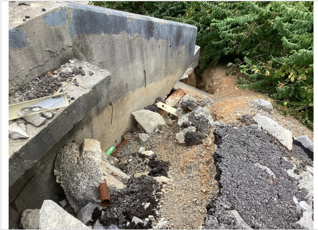
Behind wing 1 right - Heavy erosion (15'Lx4'Wx4'H)
