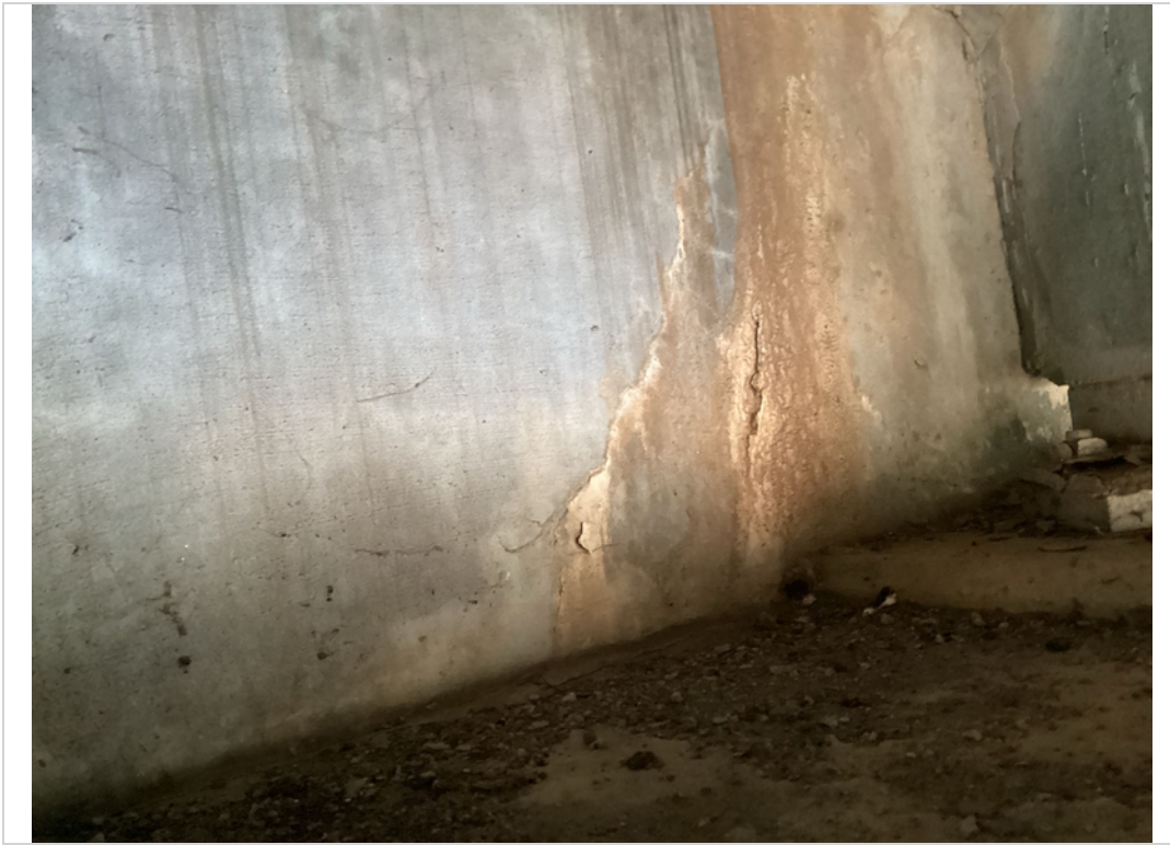
Backwall abutment 1 - Hairline cracks w/ leaching ((Typical abutment 2)
