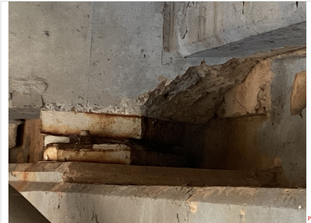
Span 1 Beam B - Spall behind bearing area (1'L x 1'H x 1"D)
