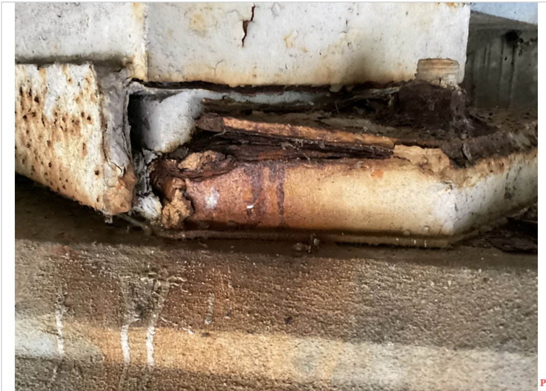
Span 1 Bearing D left - moderate corrosion (Typical A - D)
