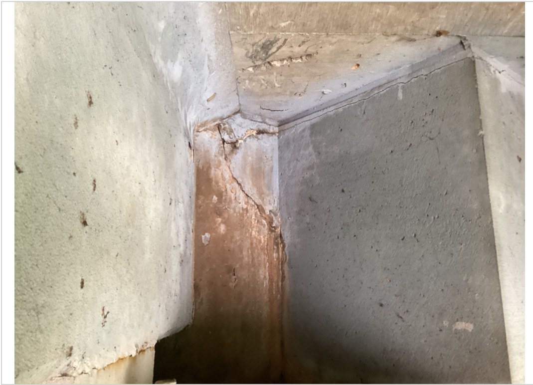
Abutment 2 backwall at Beam D right - cracks up to 1/8" with leaching
