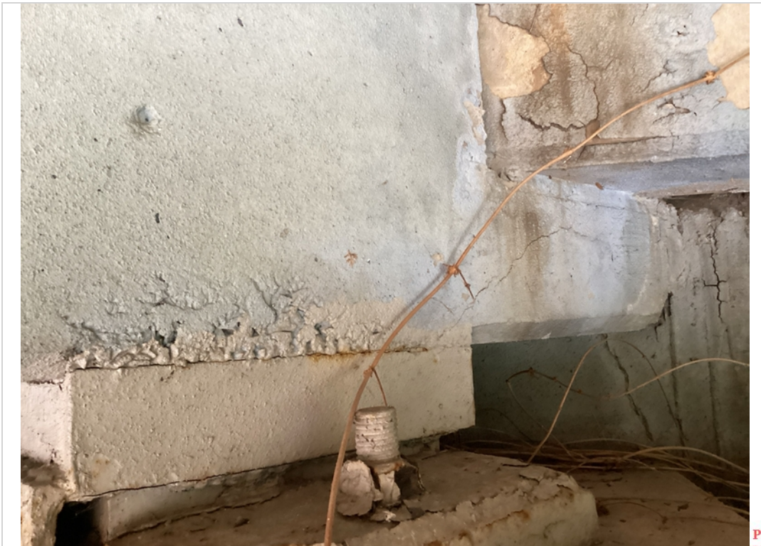
Span 3 Beam D behind bearing area - Hairline crack
