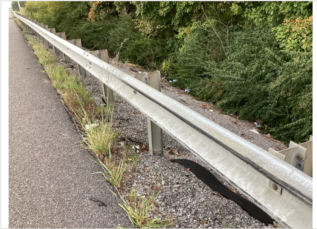
Approach 1 right rail - scrapes
