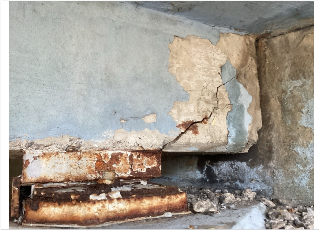
Span 1 Beam A - Spall in place behind bearing area (1'L x 1'H x 1"D)
