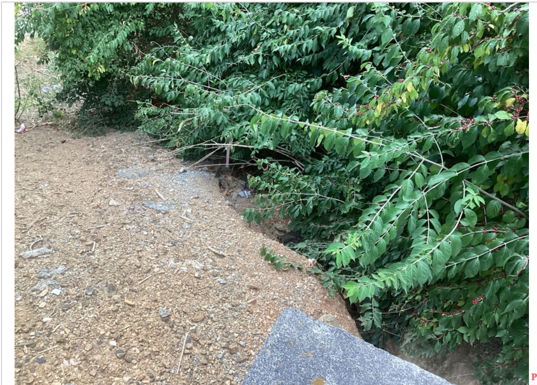
Embankment right - Erosion channel (10'Lx18"Wx3'D)
