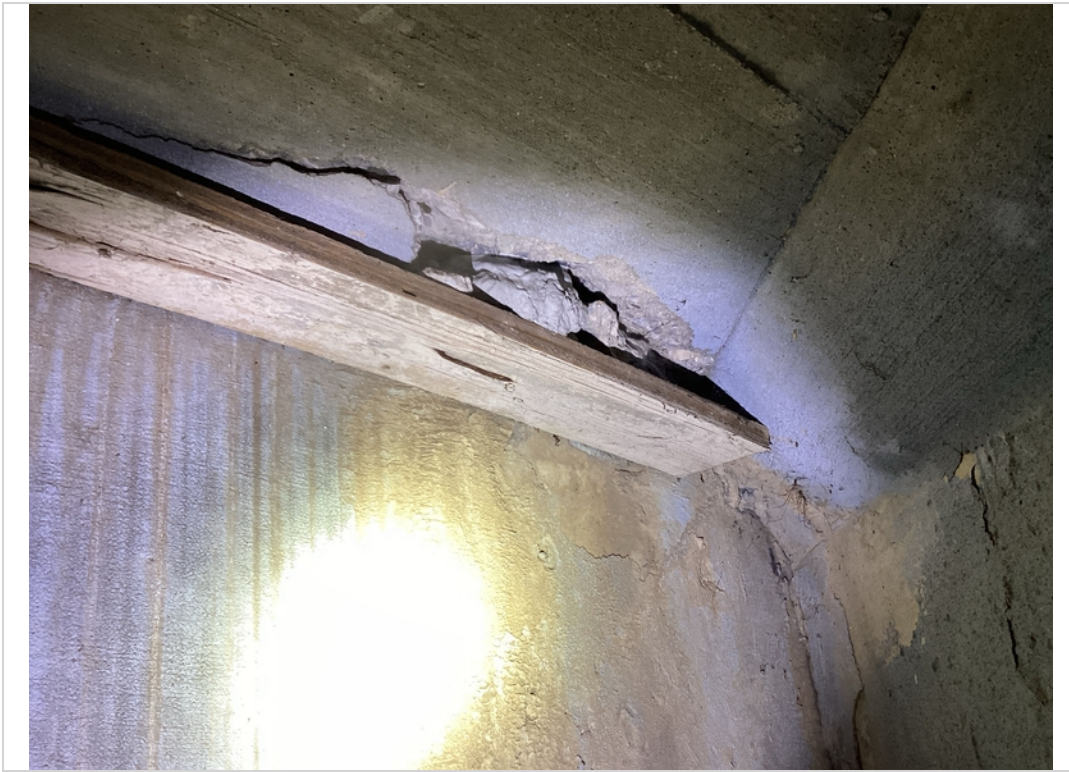
Span 1 Bottom deck at Beam D right - Spall with exposed rebar (1'W x 6"L x 3"Dp)
