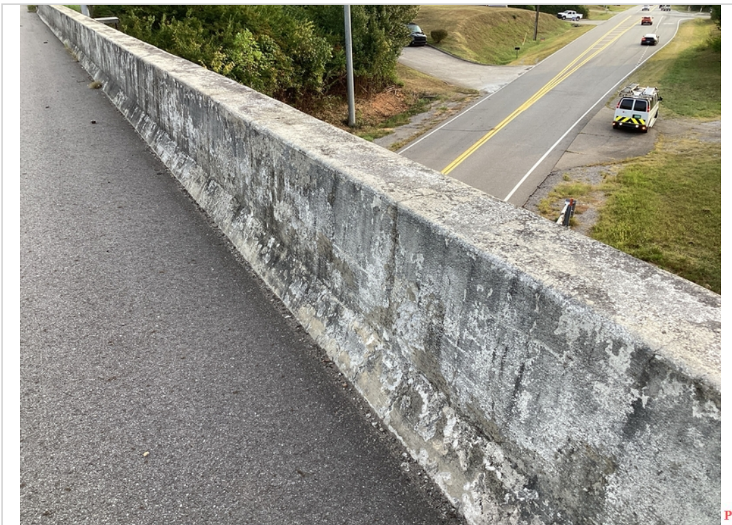
Deck 2 right rail - texture coat scaling (typical all)
