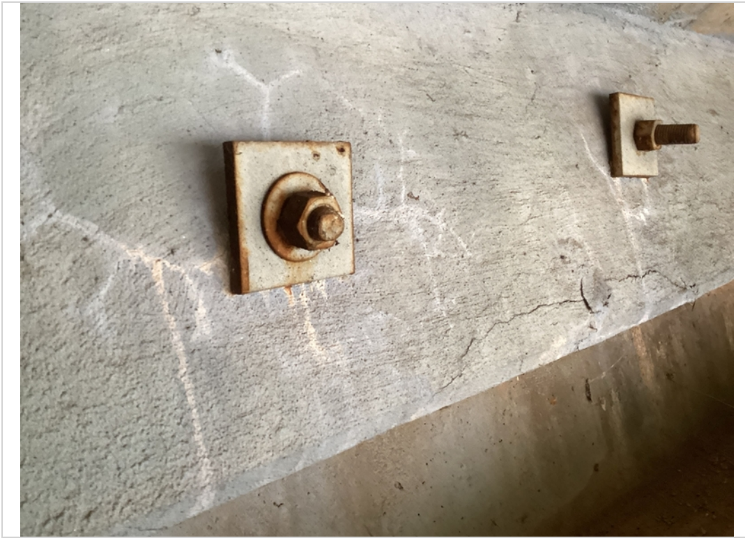
Diaphragm between beams B/C abutment 2 - Hairline map cracks (Typical abutment 1) & cracks up to 1/8"
