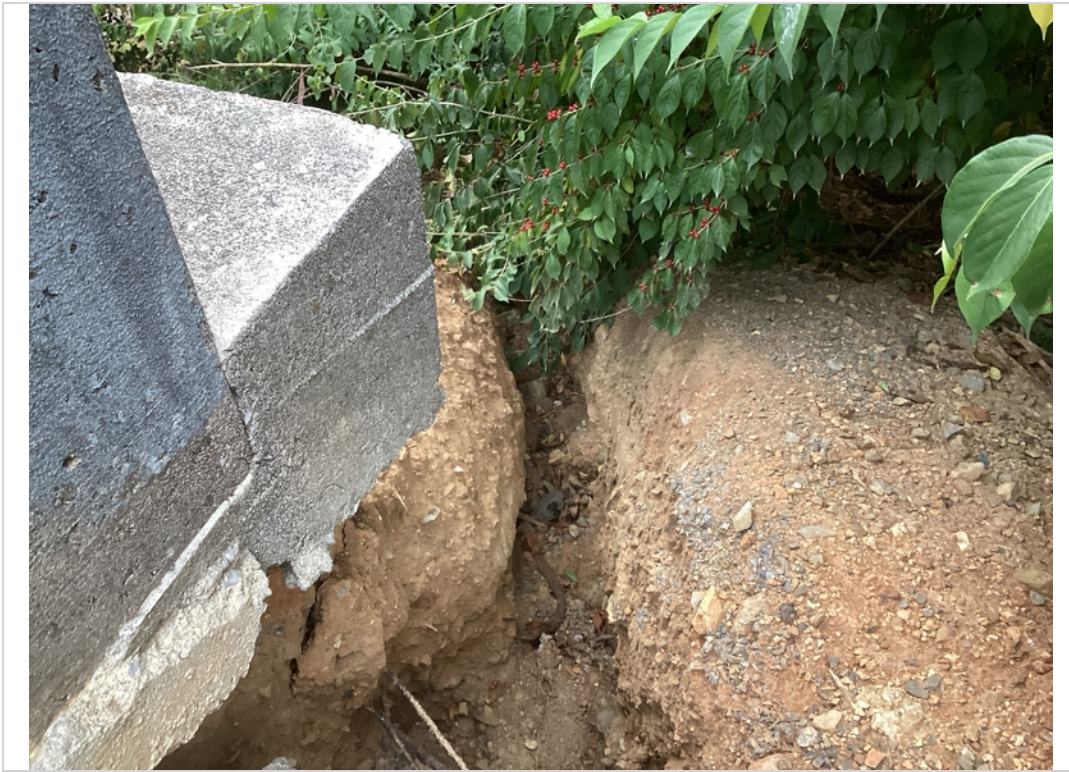
Embankment right - Erosion channel (10'Lx18"Wx3'D)
