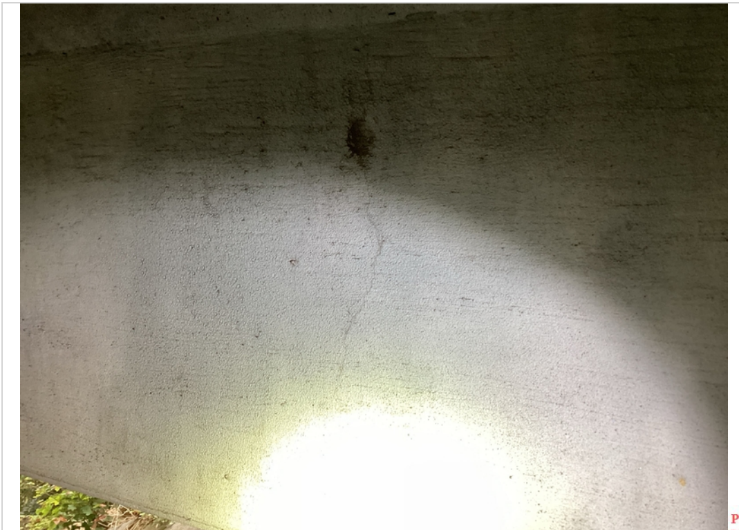
Span 1 Beam E - Hairline cracks (Typical )
