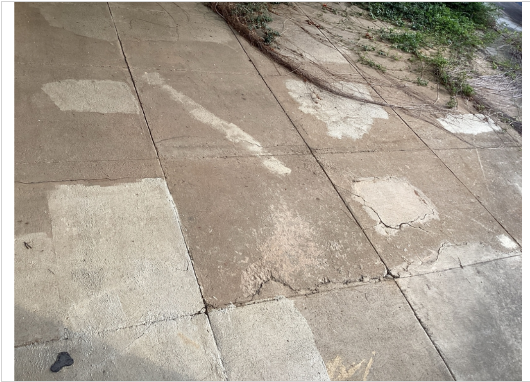
Abutment 2 concrete slope - Cracking up to 1/8"
