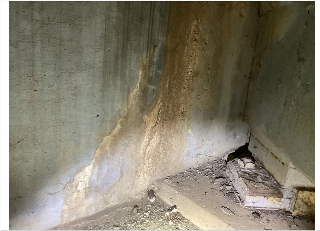
Span 1 Backwall at Beam D right - Hairline cracks with leaching
