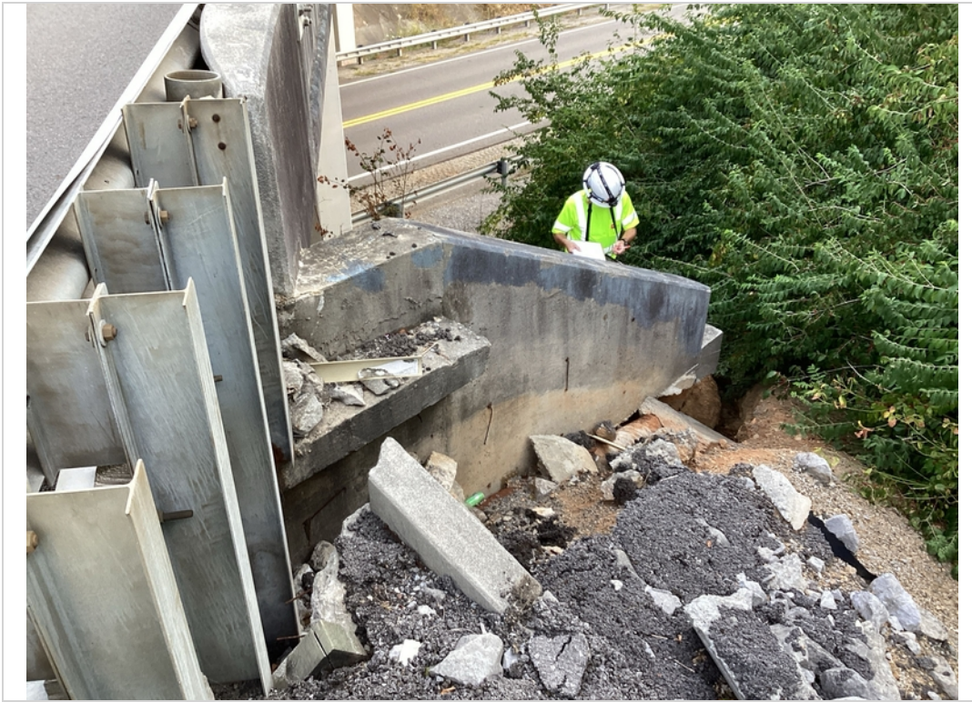
Approach 1 right embankment - erosion
