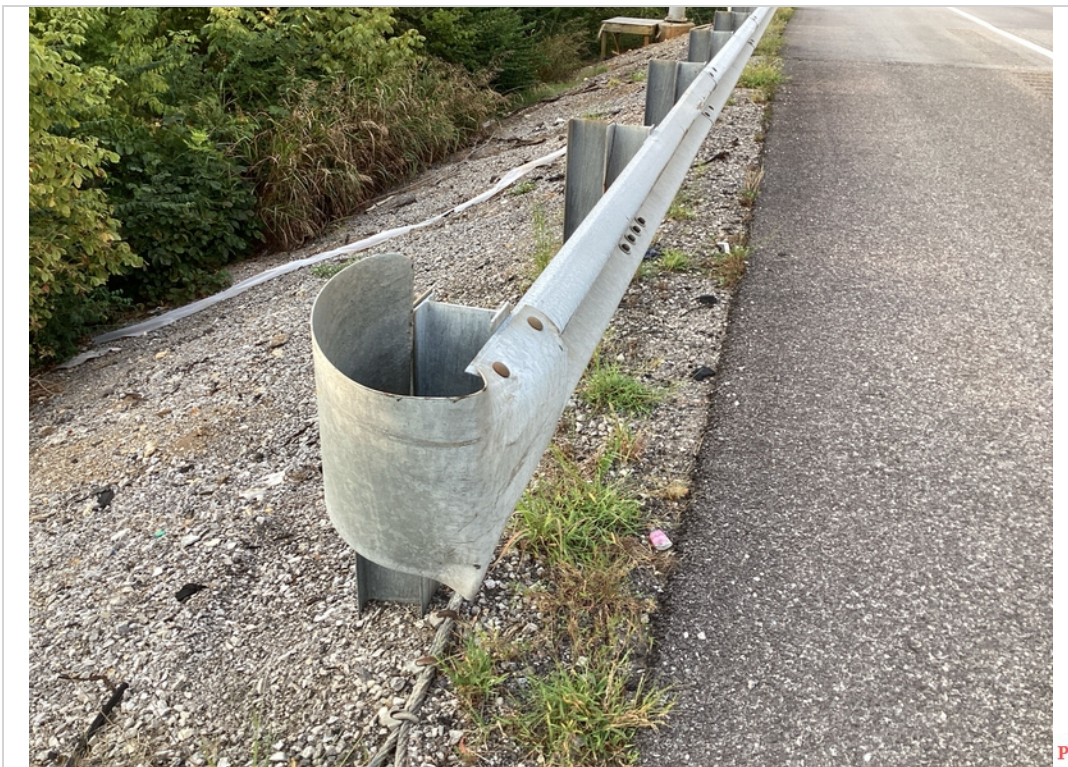
Approach 2 right terminal - minor collision damage
